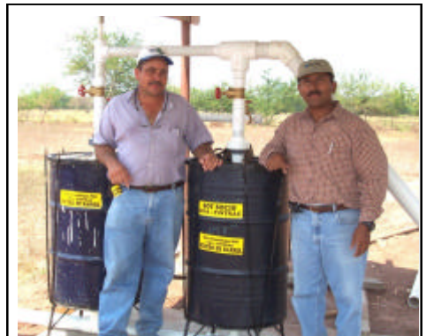
Technical representative assisting in the installation of two Fintrac/CDA designed sand filters in Comayagua
