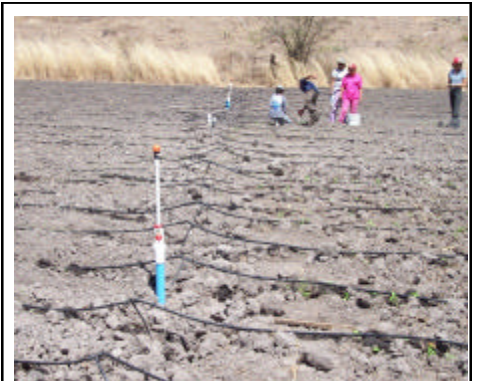
Drip irrigation system installed for jalapeño pepper production
