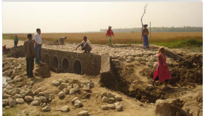
This pipe culvert is not yet complete, but it is already being used – Shripur VDC
