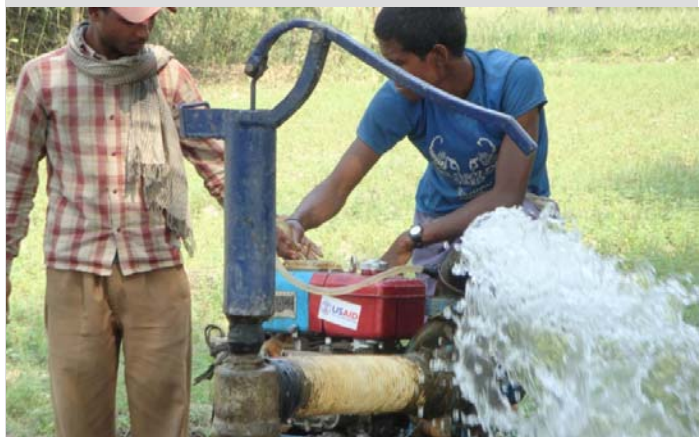
LIG trainees test their program-supported diesel pump and shallow tube well installation – Haripur VDC
