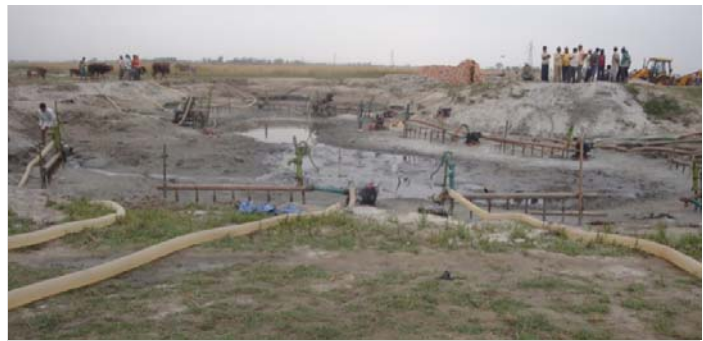
The high water table at many sites near the Koshi River requires extensive drainage before construction can begin.
