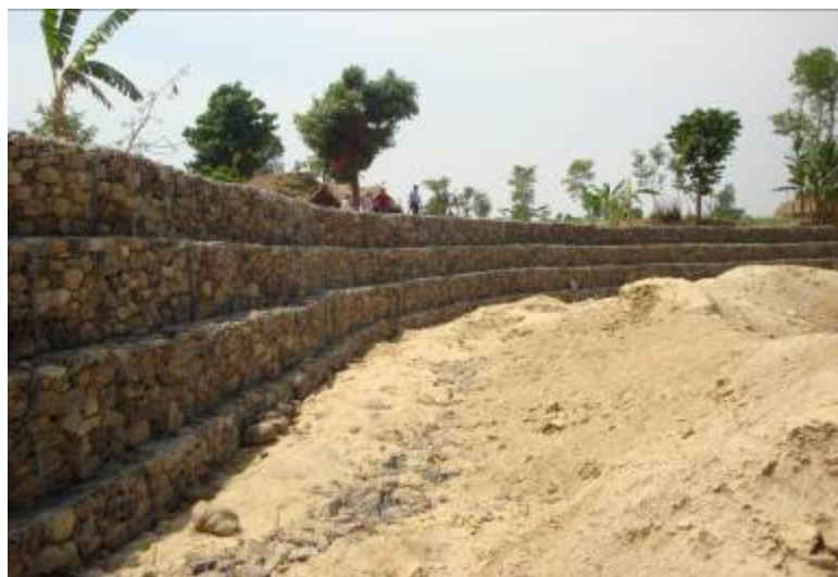
USAID-NFRP built this erosion and river control gabion in Pathariya VDC, Kailali district.
