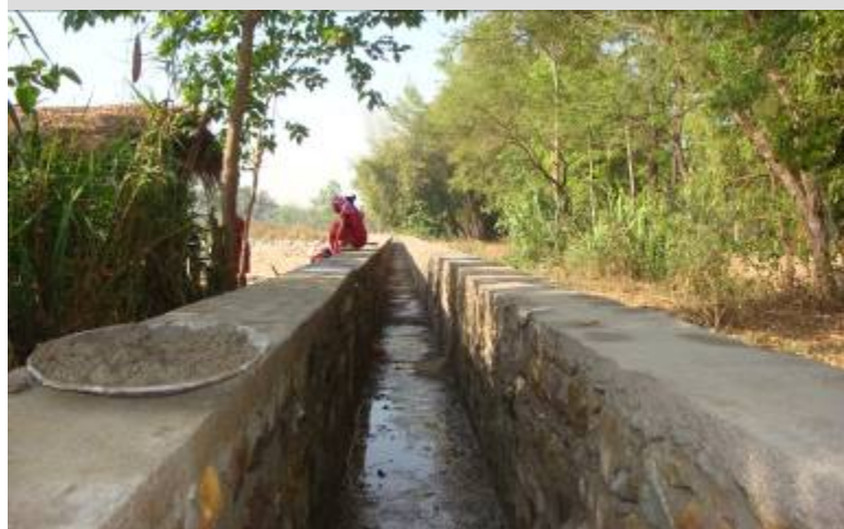
The program is improving irrigation by rehabilitating aqueducts such as this one in Thakurdwara VDC, Bardiya district.
