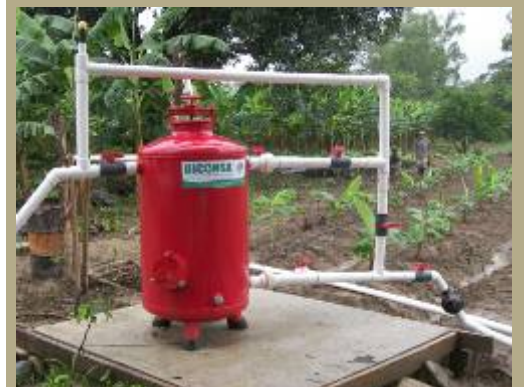
A sand filter is incorporated into the drip system.
