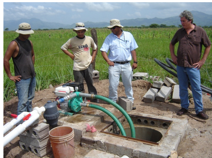
Pumping System, Visit with Fintrac's Vice President, Olancho
