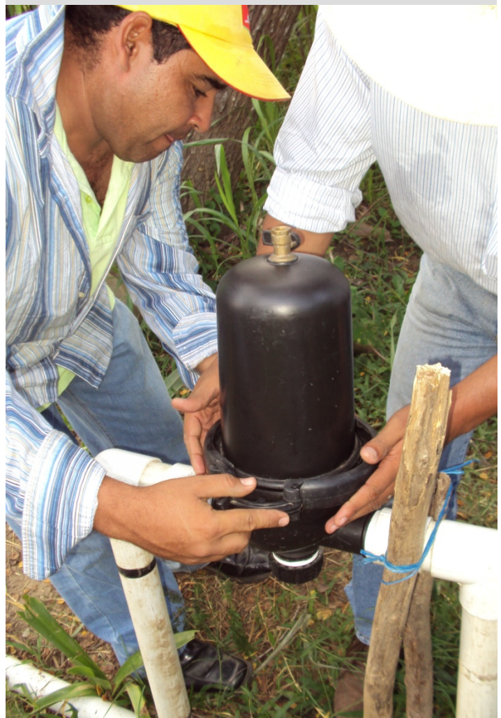
Maintenance of irrigation filter, Macuelizo, Santa Bárbara
